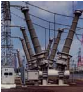
GAS switch gear (GCB/GIS)
